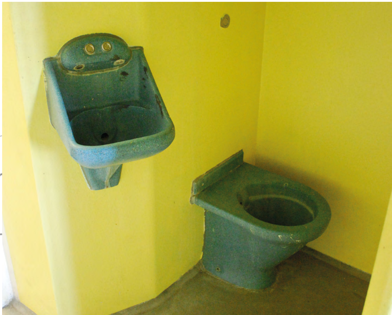
Segregation Unit toilet and sink, Colnbrook IRC
