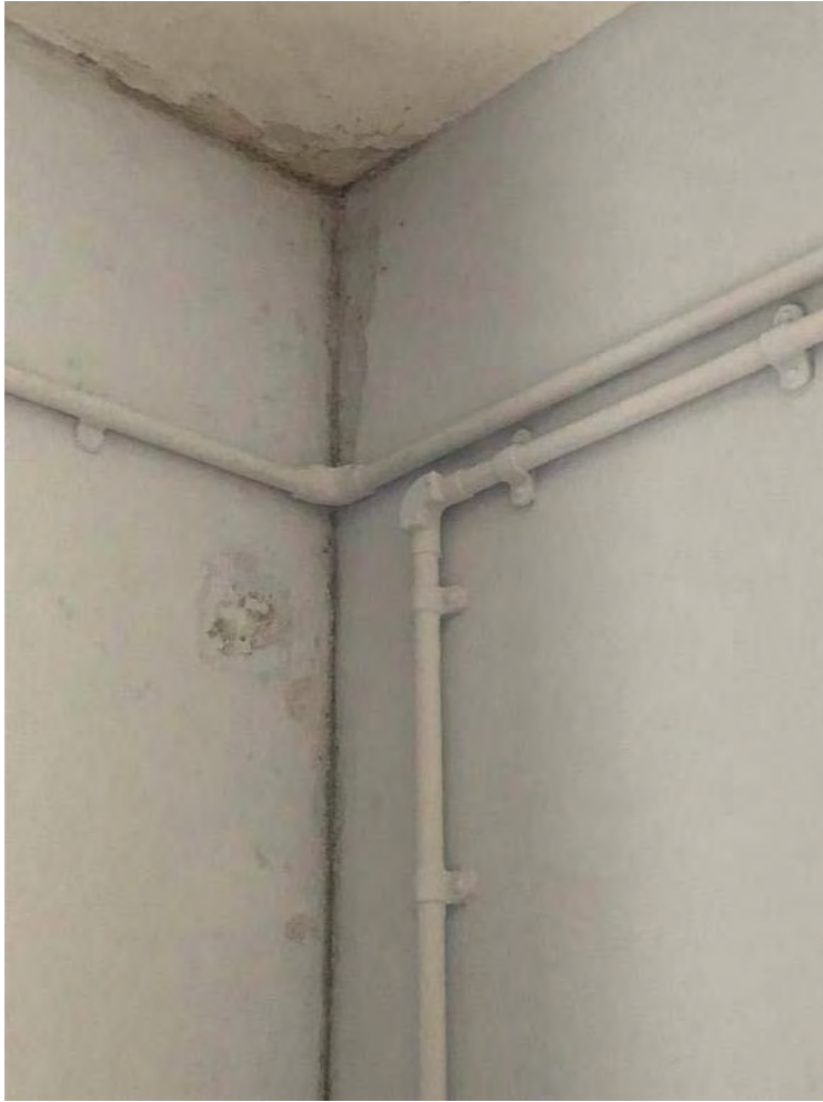
Peeling paint and damp in a room
