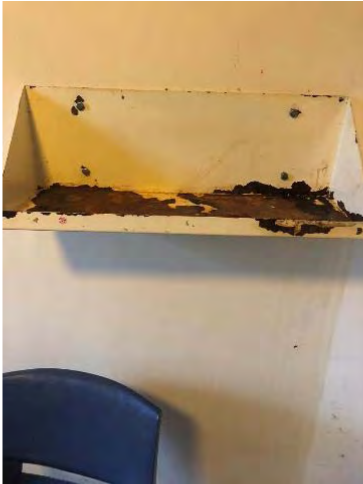
Poor condition of shelf in room
