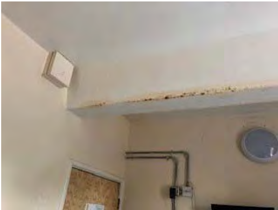
Evidence of rust or water damage in a room
