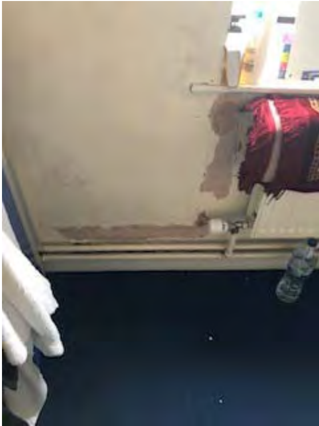
Damaged and poorly decorated wall plaster in a room
